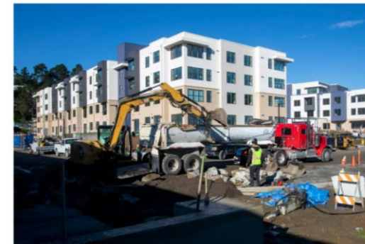
DAILY CITY, CALIFORNIA - DECEMBER 30. Construction means completion on 122 subsidized apartments for teachers and staff in the Jefferson Union High School District, Thursday, December 30, 2021. In Daily City, Calif. (Karl Menden/Bay Area News Group)
